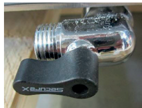
1. Control valve of steam generator
